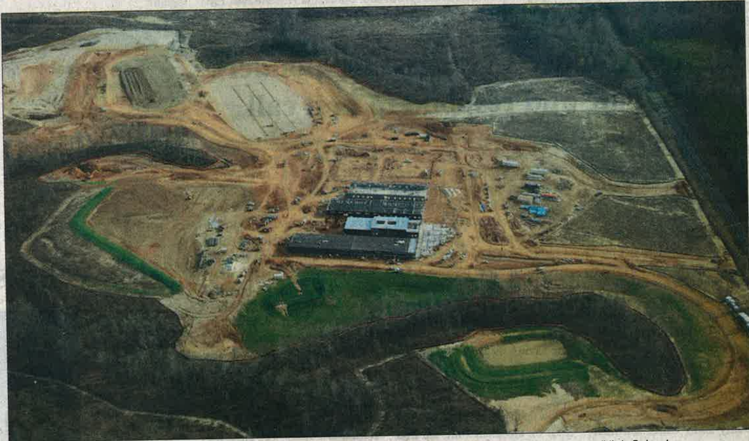
Pictured above is an aerial photo of the ongoing construction of the new Marion County Middle/High School.
